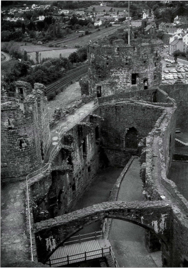
Looking down from the inner ward on to the hall complex in the outer ward of Conwy. Half the hall is provided with a narrow cellar. The stone arch is a 14th-century addition replacing the original wooden structures. Note the continuous route round the towers from the wall-walk.
