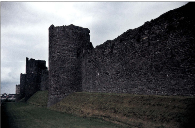
Towers 6 to 9 on Town Ditch Road in Conwy. Note the change in colour of the stonework on Tower 6 in the distance.
