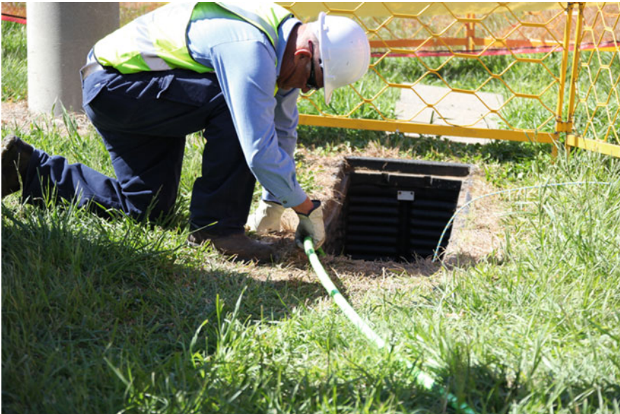
Optic fibre being installed underground. Source: Copyright © 2013 NBN Co Limited. All rights reserved 104
