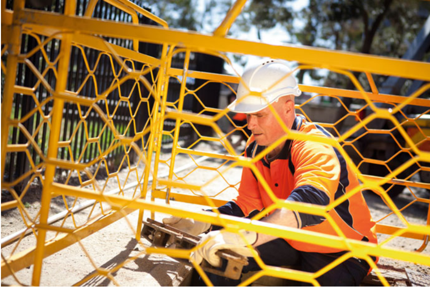
Optic fibre installation underground. Source: Copyright © 2013 NBN Co Limited. All rights reserved 108
