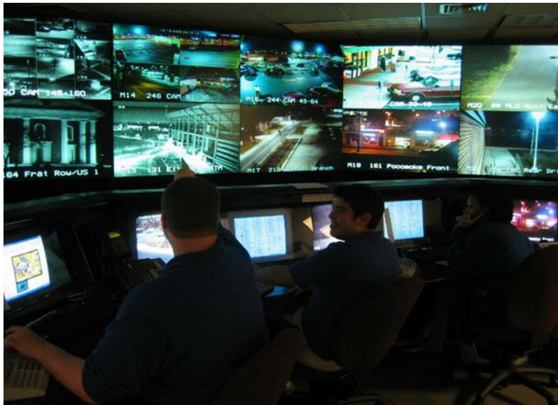
FIGURE 5.5 A typical security operations center
